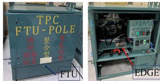
Figure 2. The desired EDGE platform inside the TPC's FTU chassis.
